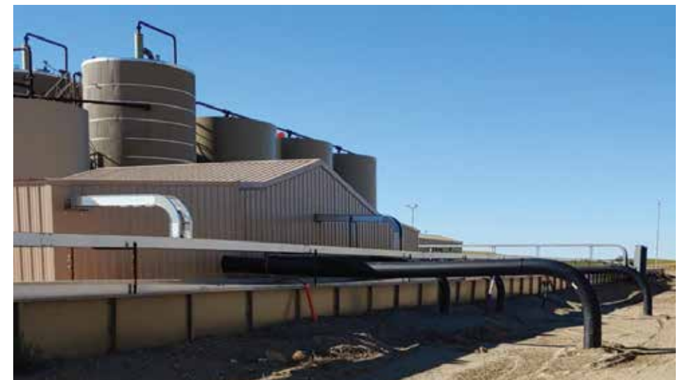
Figure 3: Produced Water Mains Entering a Typical Cleaning and Injection Facility
