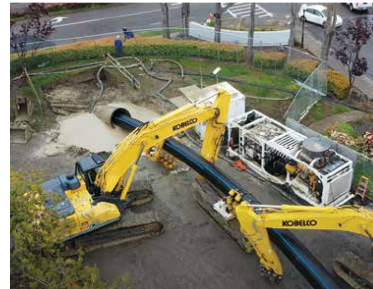
Figure 2: Fused 32-inch diameter PE4710 pipe string on rollers being pulled to borehole
